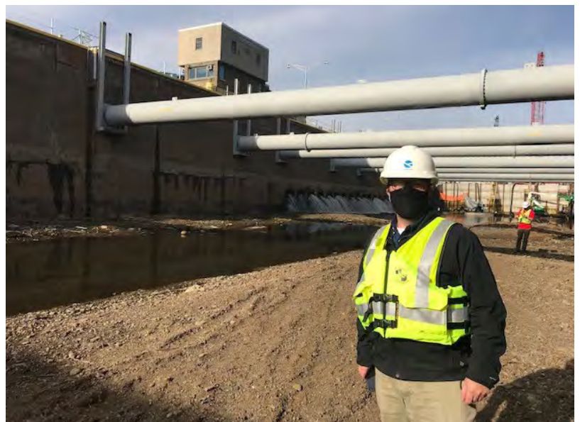
Matt inside dewatered Emsworth chamber -- October 14, 2020
